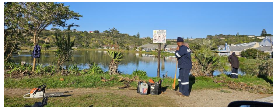
NM MAINTENANCE TEAMS IN OPERATION AT DUCK POND PORT ALFRED (source: TMRP)
